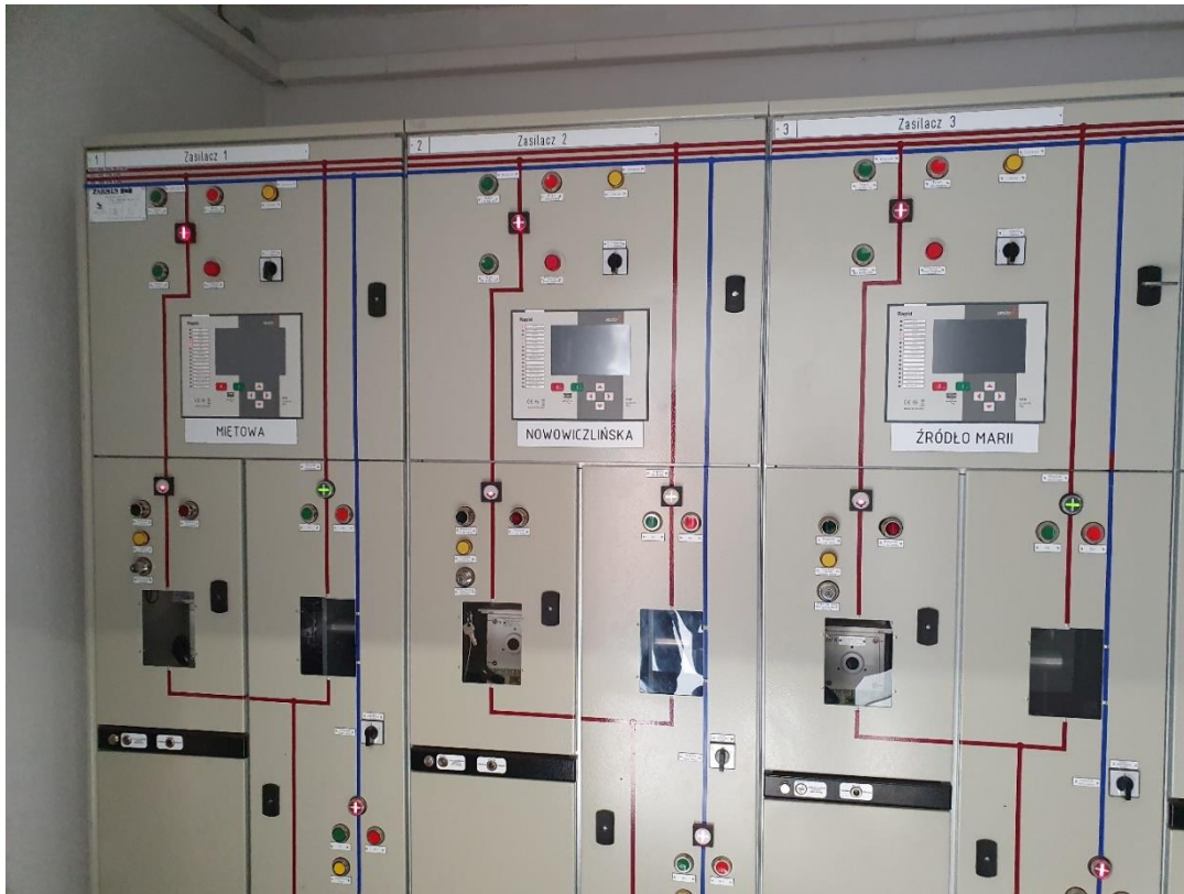
Figure 6. Diagram of the substation and the cabinet with power devices of the Nowowiczlińska substation.
