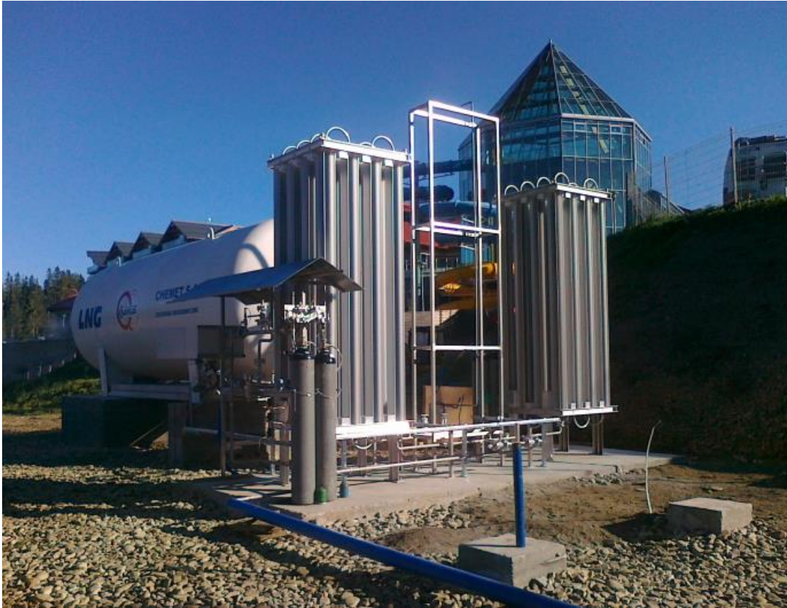
Figure 12. Chemet S.A. LNG regasification station [16]
