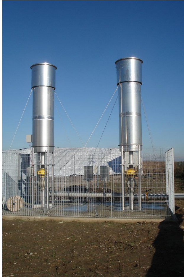
Figure 15. Torches for burning biogas in the biogas plant ( www.aat-biogas.at )
