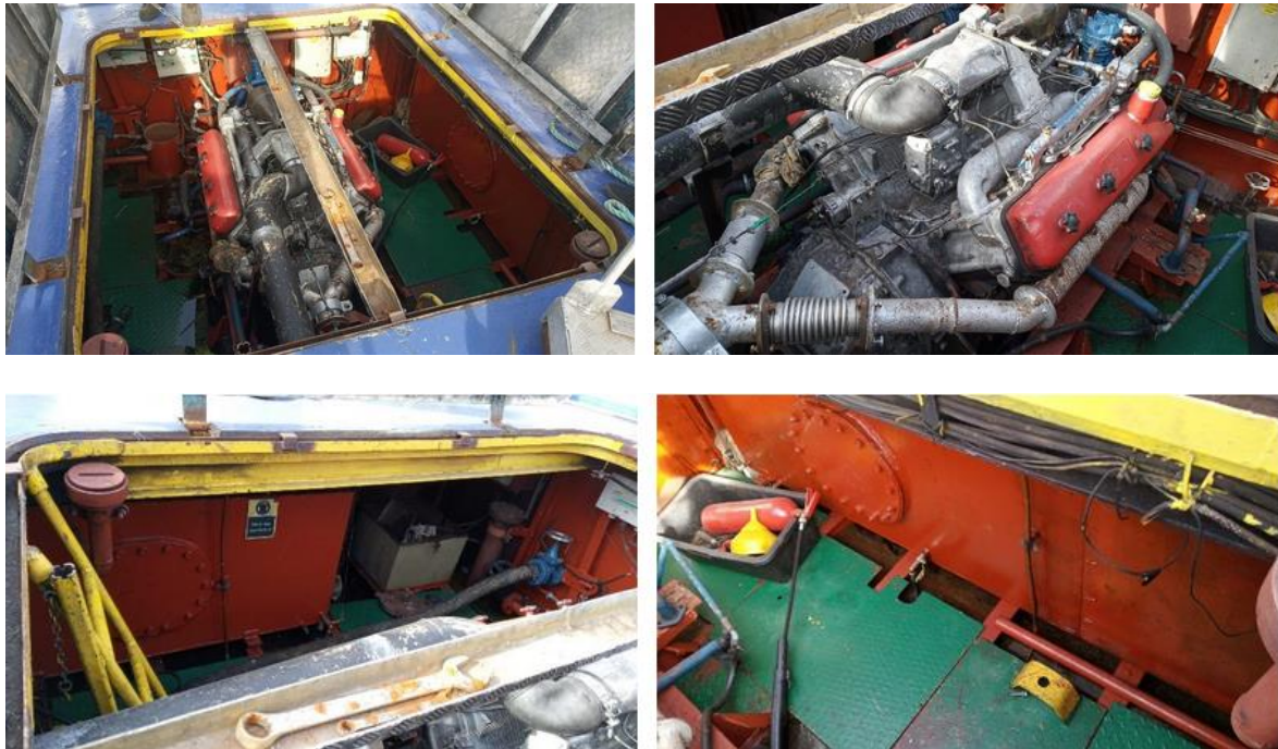
Figure 26. View of the engine room from the deck perspective after opening the hatch and a view of the fuel tanks on each side.
