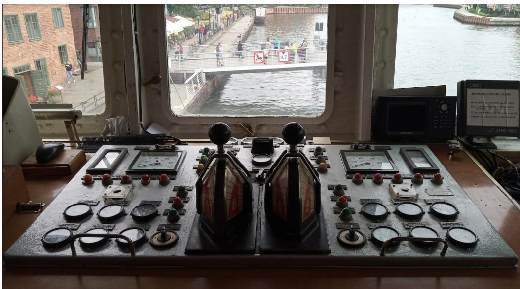
Figure 22. Emergency control panel with measuring indicators.
